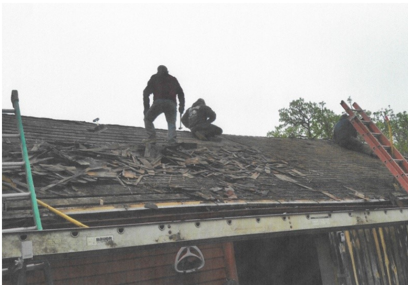
Summer 2019 roof replacement (this roof had 2 layers of asphalt shingles over cedar shakes)
